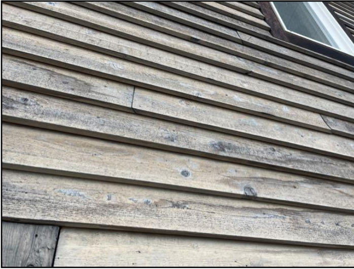
Paint or stain - needed
