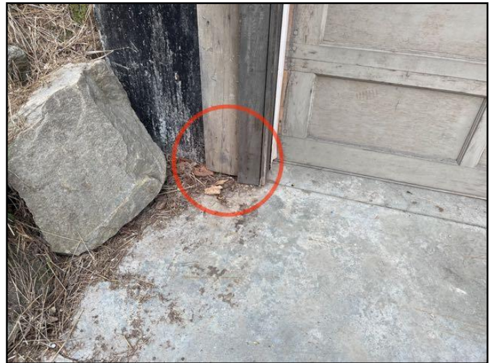
Too close to grade
