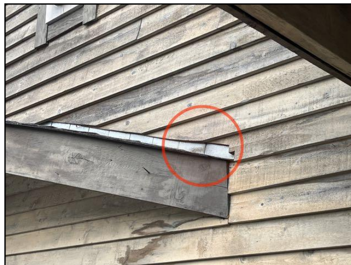
Kickout flashing - missing
