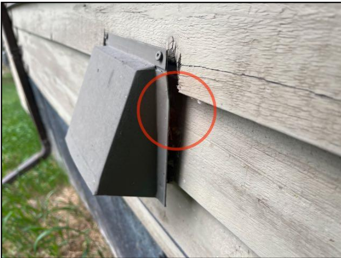
Caulking missing or ineffective
