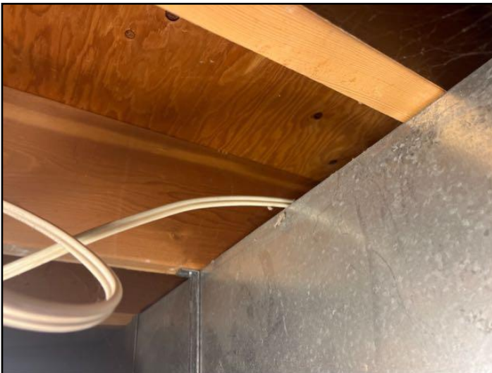
Wires noted touching duct work. Should the...
