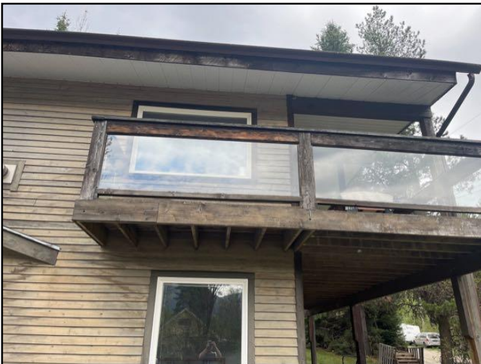
Paint or stain needed
