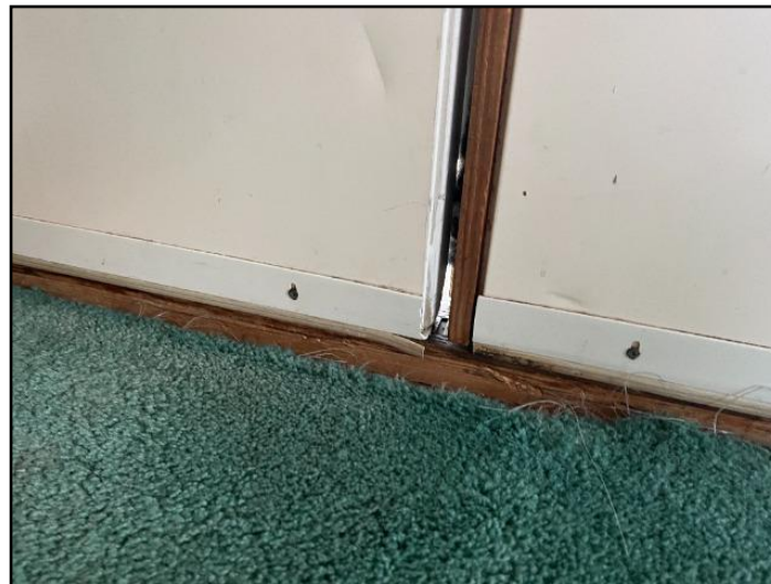
Loose or poor fit
