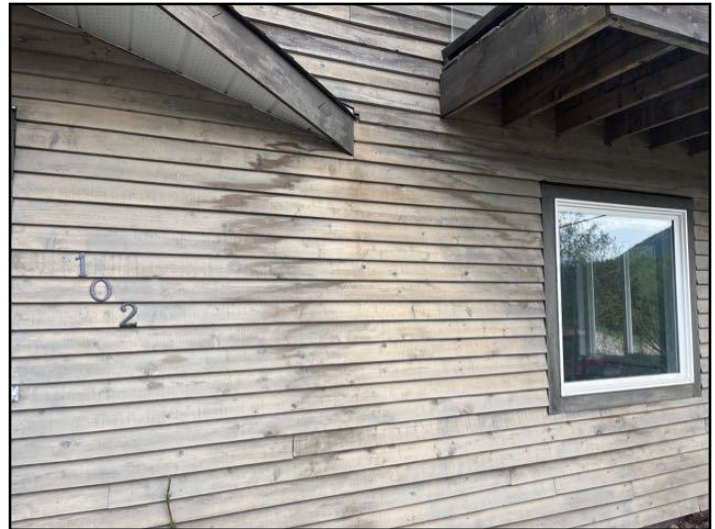
Kickout flashing - missing
