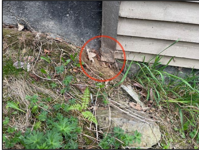
Too close to grade
