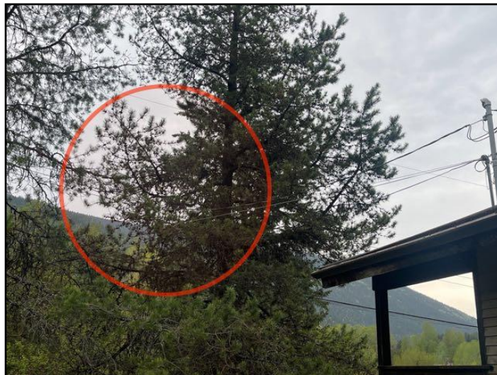
Branches / vines interfering with wires
