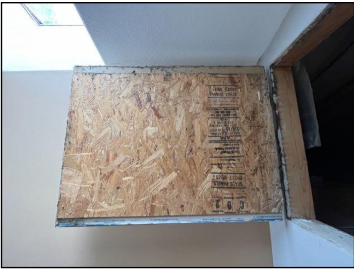
Not insulated and not weatherstripped
