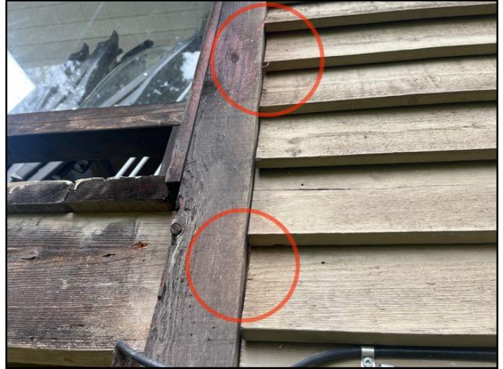
Caulking missing or ineffective
