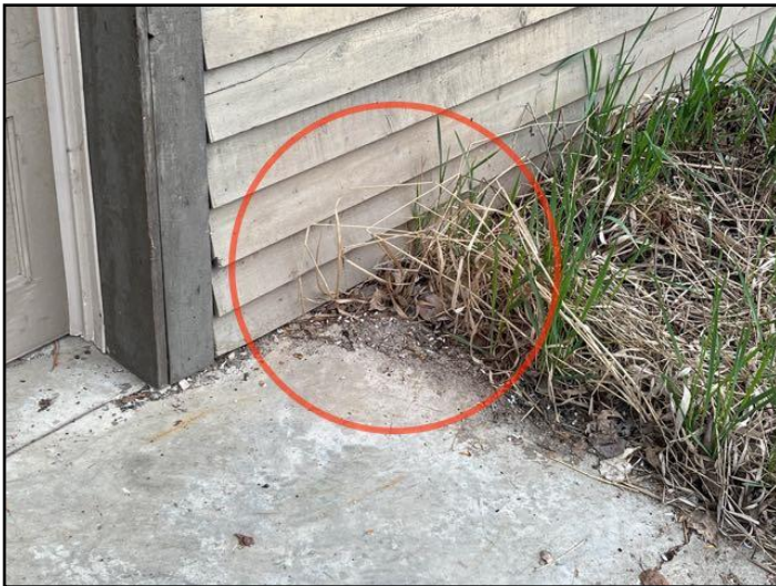
Too close to grade
