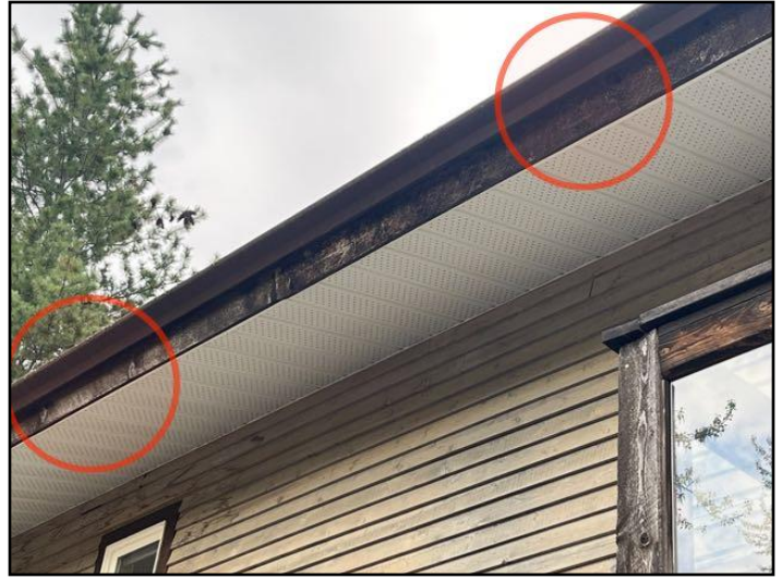
Paint or stain - needed
