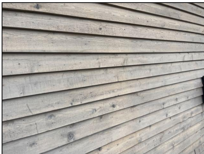
Paint or stain - needed
