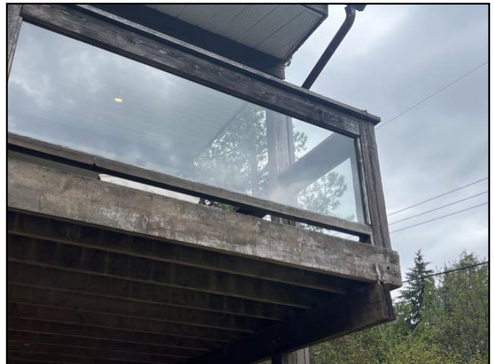
Paint or stain needed
