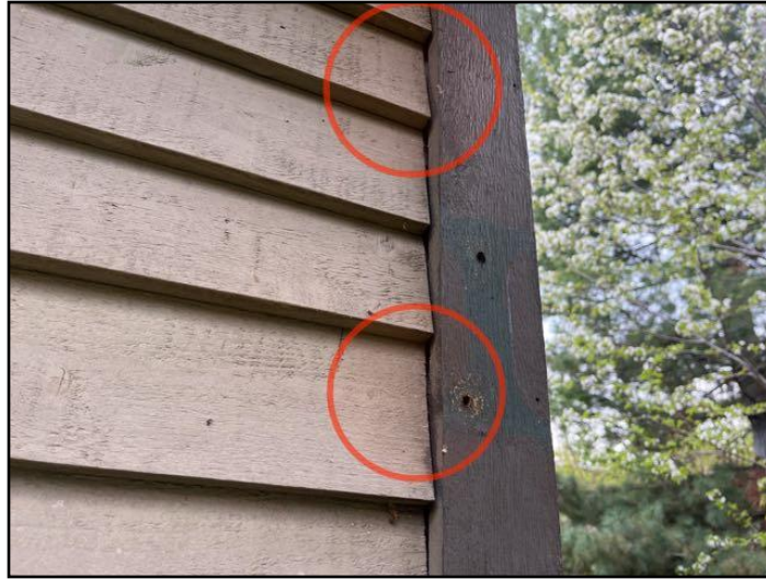
Caulking missing or ineffective
