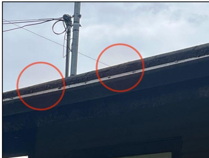
Loose or damaged
