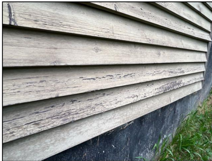
Paint or stain - needed
