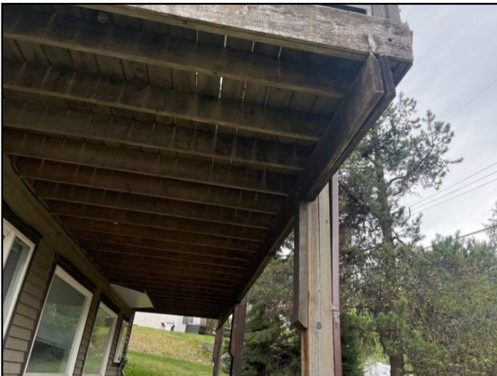
Poor post connection
