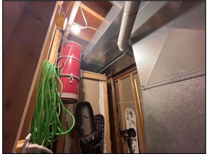
not gas tight
