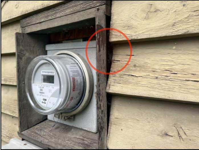
Caulking missing or ineffective
