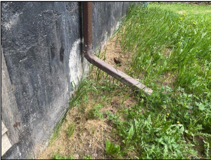
Discharge too close to building
