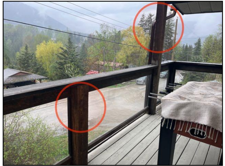
Paint or stain needed
