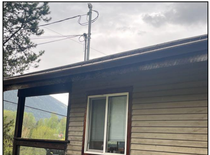
Loose or damaged
