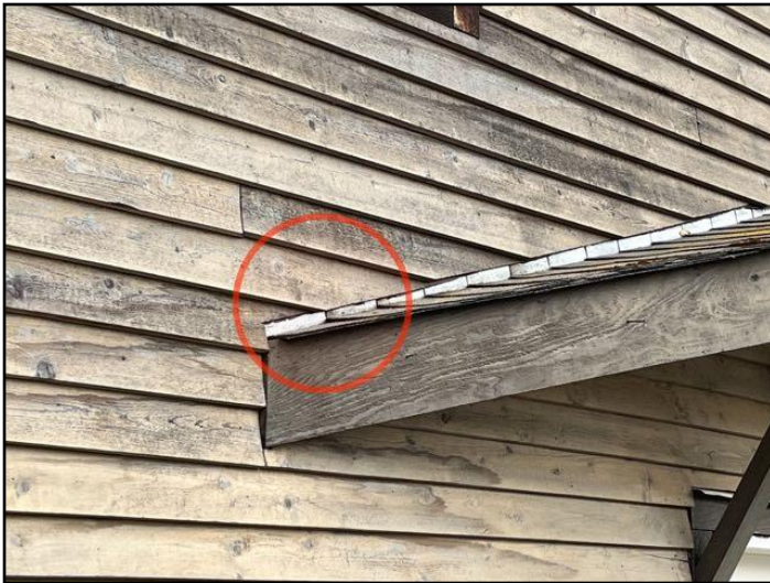
Kickout flashing - missing
