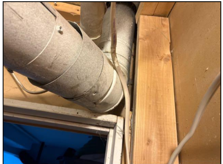
Contacting the furnace vent pipe (high heat)
