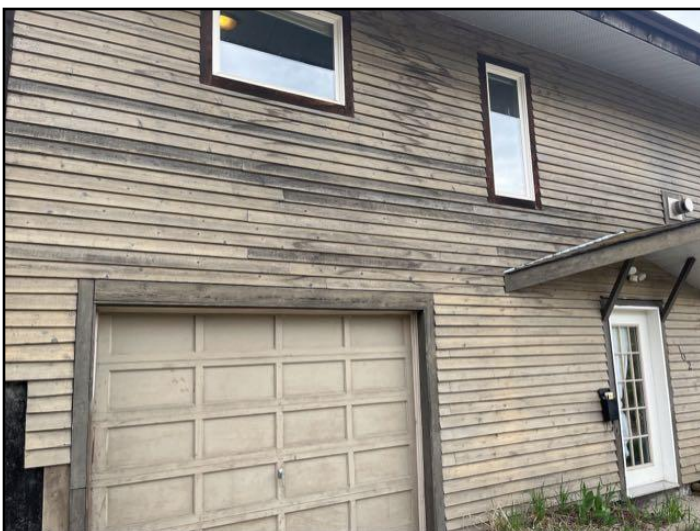
Paint or stain - needed
