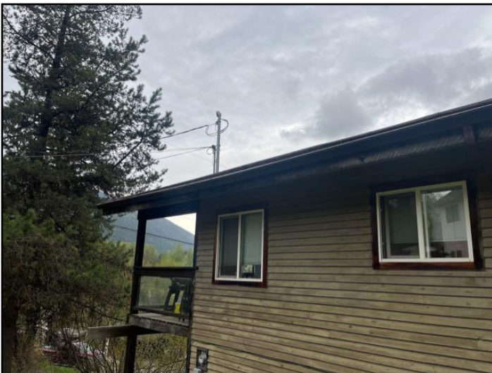
Loose or damaged
