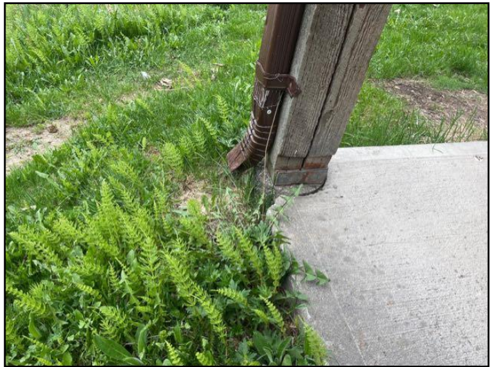
Discharge too close to building
