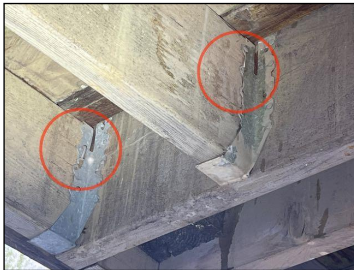
Poor end bearing, joist hanger connections
