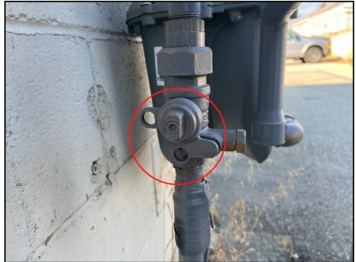
Main shut off
