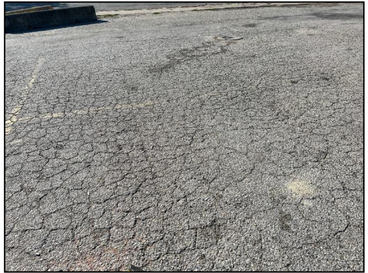
Local surface deterioration
