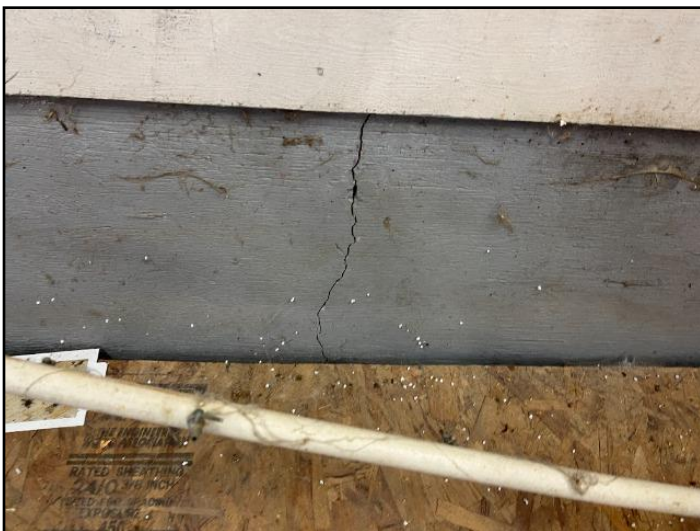
Settlement cracks noted
