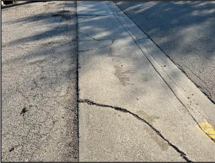
Local surface deterioration
