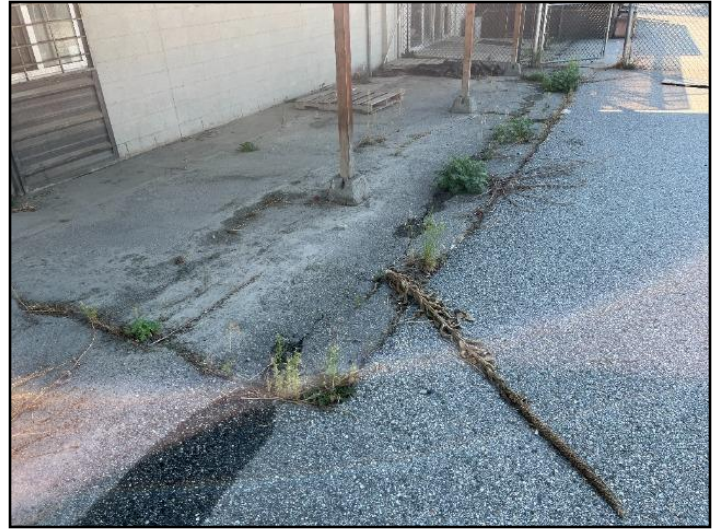
Local surface deterioration
