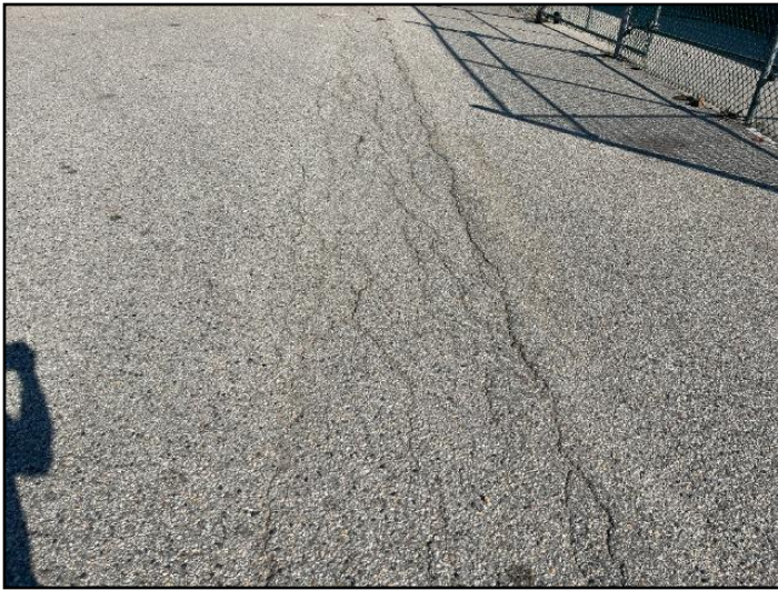
Local surface deterioration
