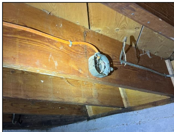
Missing on switches, outlets and junction...
