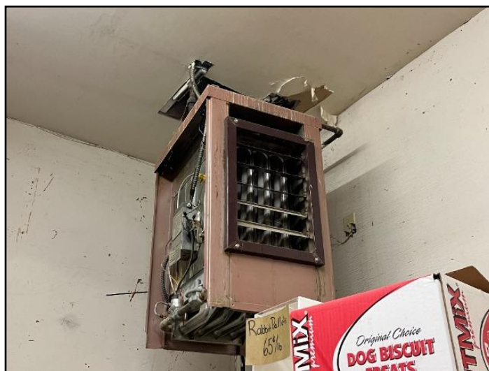
Gas-fired, unit heater
