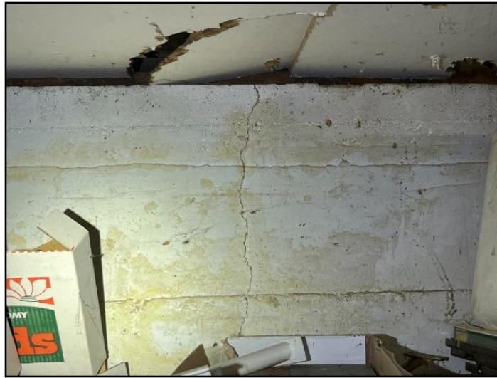
Settlement cracks noted
