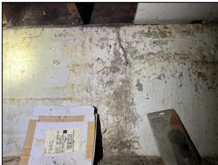
Settlement cracks noted
