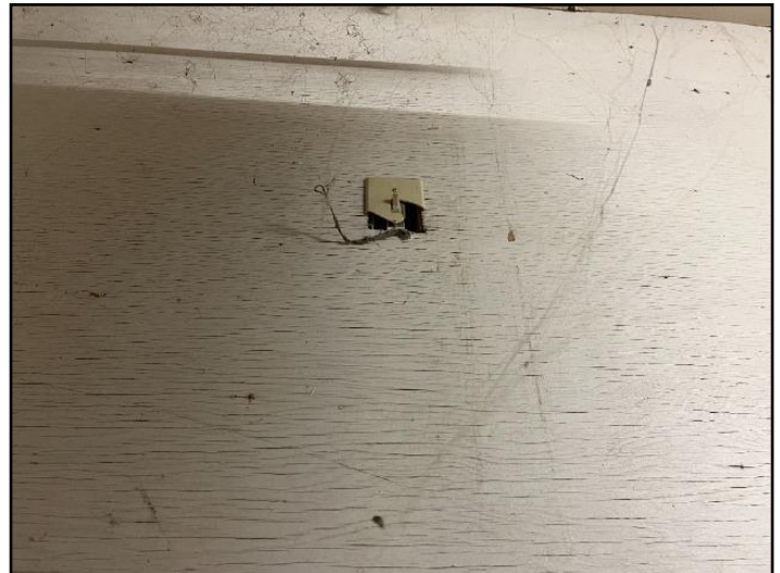
Missing on switches, outlets and junction...
