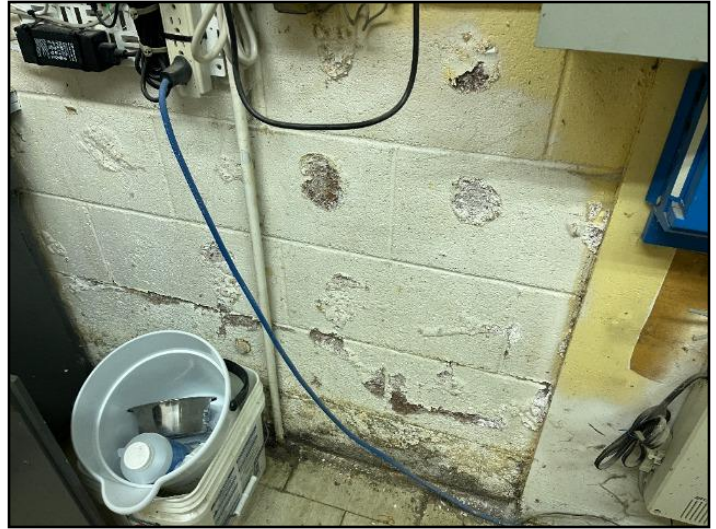
Moisture penetration/damage on interior
