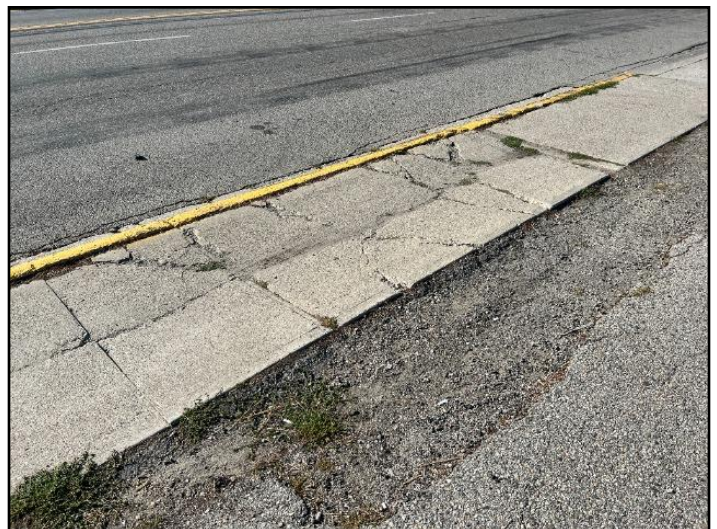
Local surface deterioration
