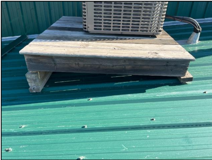
Missing vibration dampeners
