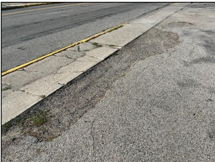
Local surface deterioration
